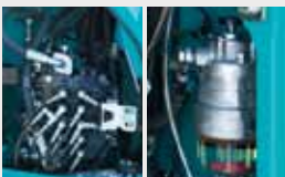
Control valve/water separator
